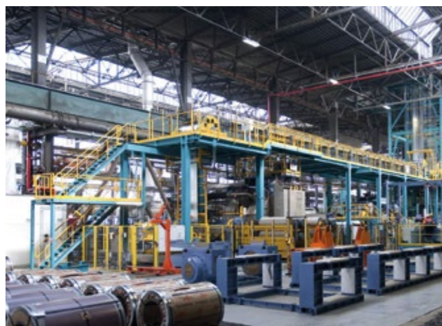
Complete in-line skin pass mill and post treatment section for automotive applications at ArcelorMittal Eisenhüttenstadt
