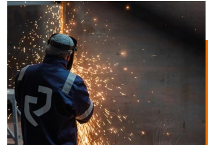
John Cockerill's global servicing & spares offer provides comprehensive maintenance programs, including preventive and regular maintenance or small revamping jobs
